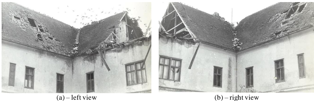
Figure 13: Failure mechanisms observed in the internal court of the case study building [16].
