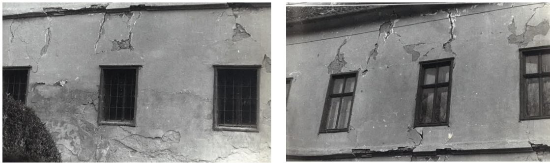
Figure 12: Vertical and diagonal shear cracks detected in the South façade of the case study building [16].
